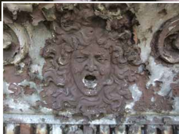
Closeup of the brownstone façades' deterioration prior to the restoration.
